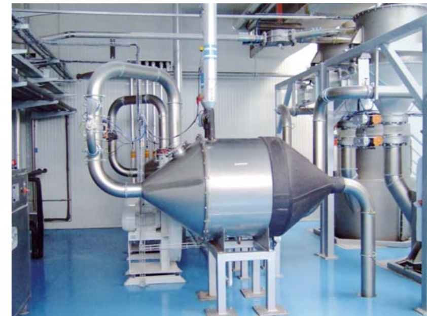
Flour cooling system
